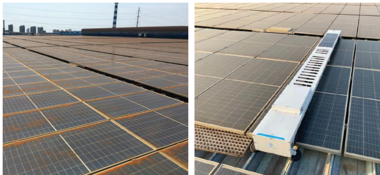
Figure (1): The Modules on the Rooftop PV Plant were Covered with Metallic Dust, Leading to Rusting. Regular Cleaning by Robots Significantly Improved the Situation of the Modules – Source: Sunpure
