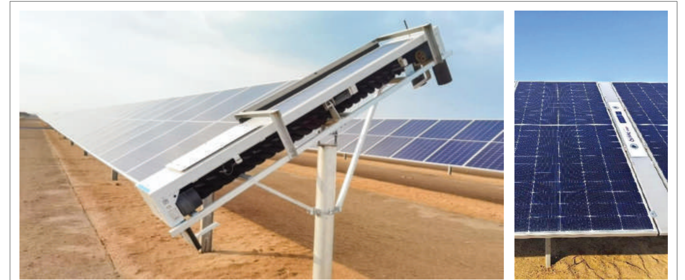
Figure (2): Robots Working on the Modules While the DustIQ Examines their Efficiency – Source: Sunpure
